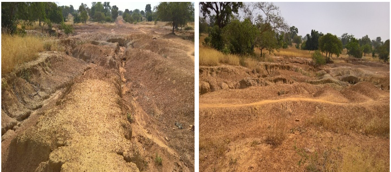
Plate 4-4: Deep gully erosion observed close to project site
